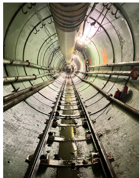
Inside the 715m long tunnel. You can see the tracks that the spoil is removed on.
