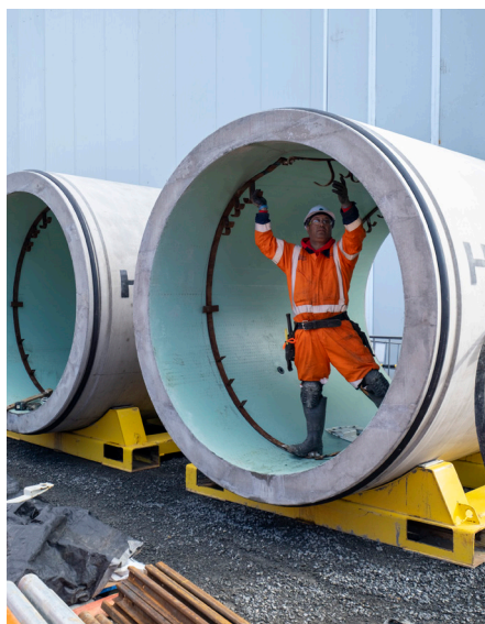
Concrete pipes being prepared to be installed into the shaft and form the link sewer.
