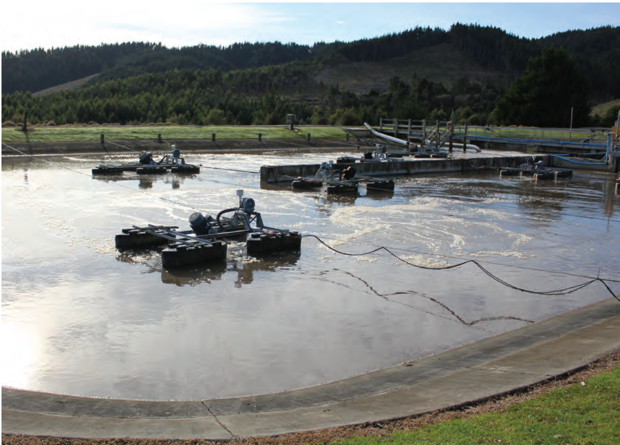
Beachlands Wastewater Treatment Plant
