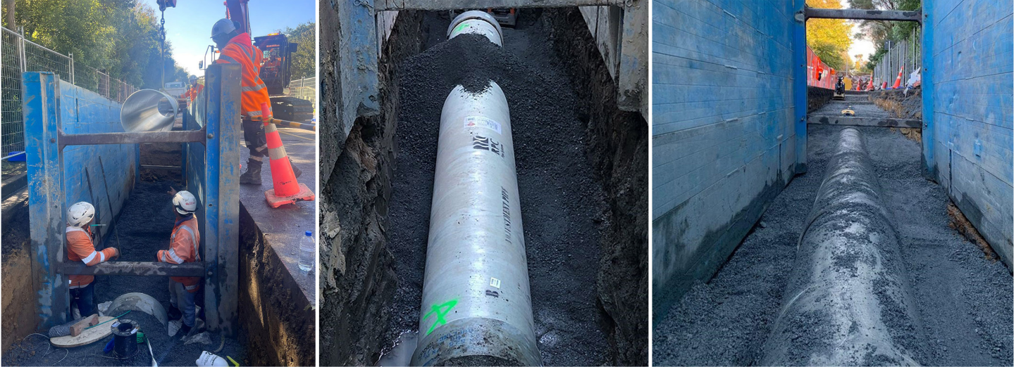
Open trench construction - a section of the new wastewater pipe has been laid and completed in the trench.
