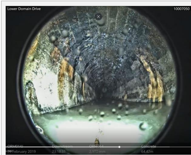
Mass ingress at block/concrete joint at 3 and 9 o'clock of CH: 64.42m
