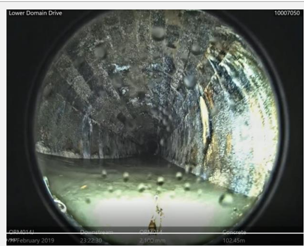
Mass ingress at block/concrete joint at 3 o'clock of CH: 102.45m
