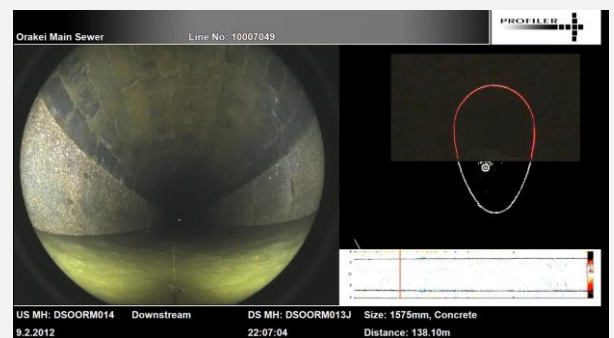
Spalling/reinforcing at 3 o'clock of CH:138.1m
