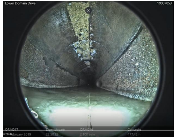
Spalling and rebar exposed at the obvert from CH:444.48m to 487.68m
