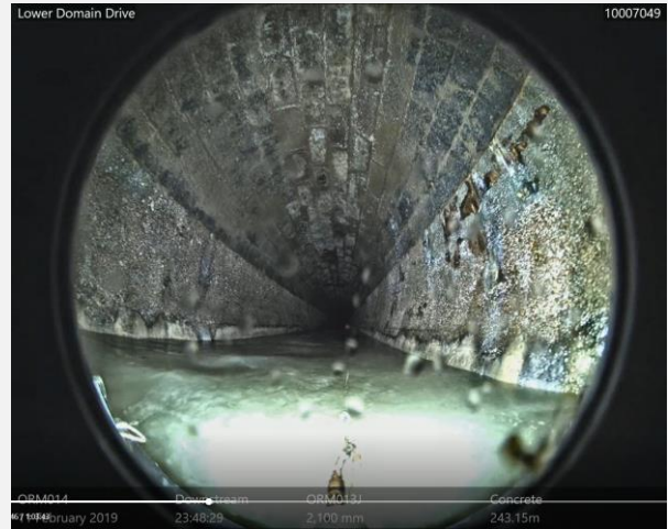
Mortar missing at 3 o'clock of CH: 243.15m
