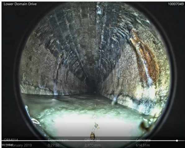
Hole/opening in blocks resulting in mass infiltration/ ingress at 3 o'clock of CH: 614.91m
