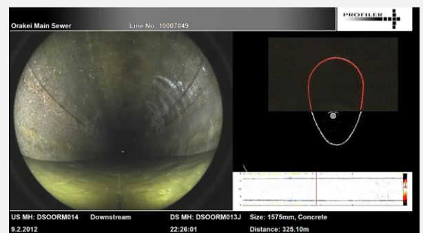
Lime leaching through the mortar is evident throughout the conduit at 3 o'clock
