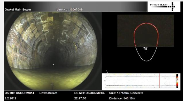
Lime leaching through the mortar is evident throughout the conduit from 9 to 3 o'clock
