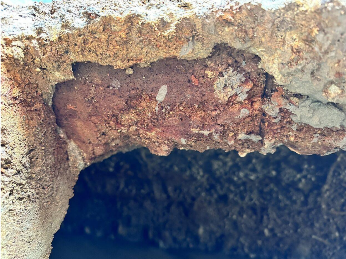
Figure 7 Weak blockwork in-situ
