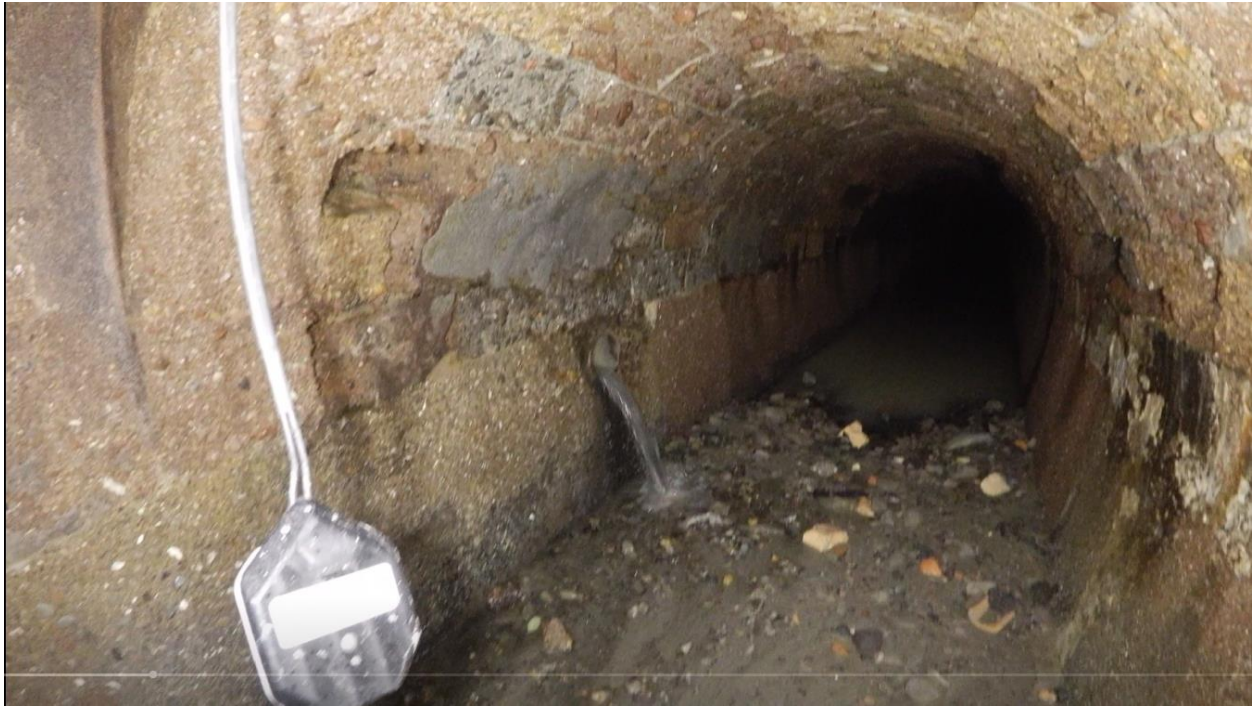
Figure 1 – Missing blocks adjacent to Manhole 15 (view is looking upstream)
