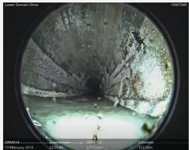
Mortar missing at 3 o'clock of CH: 312.28m
