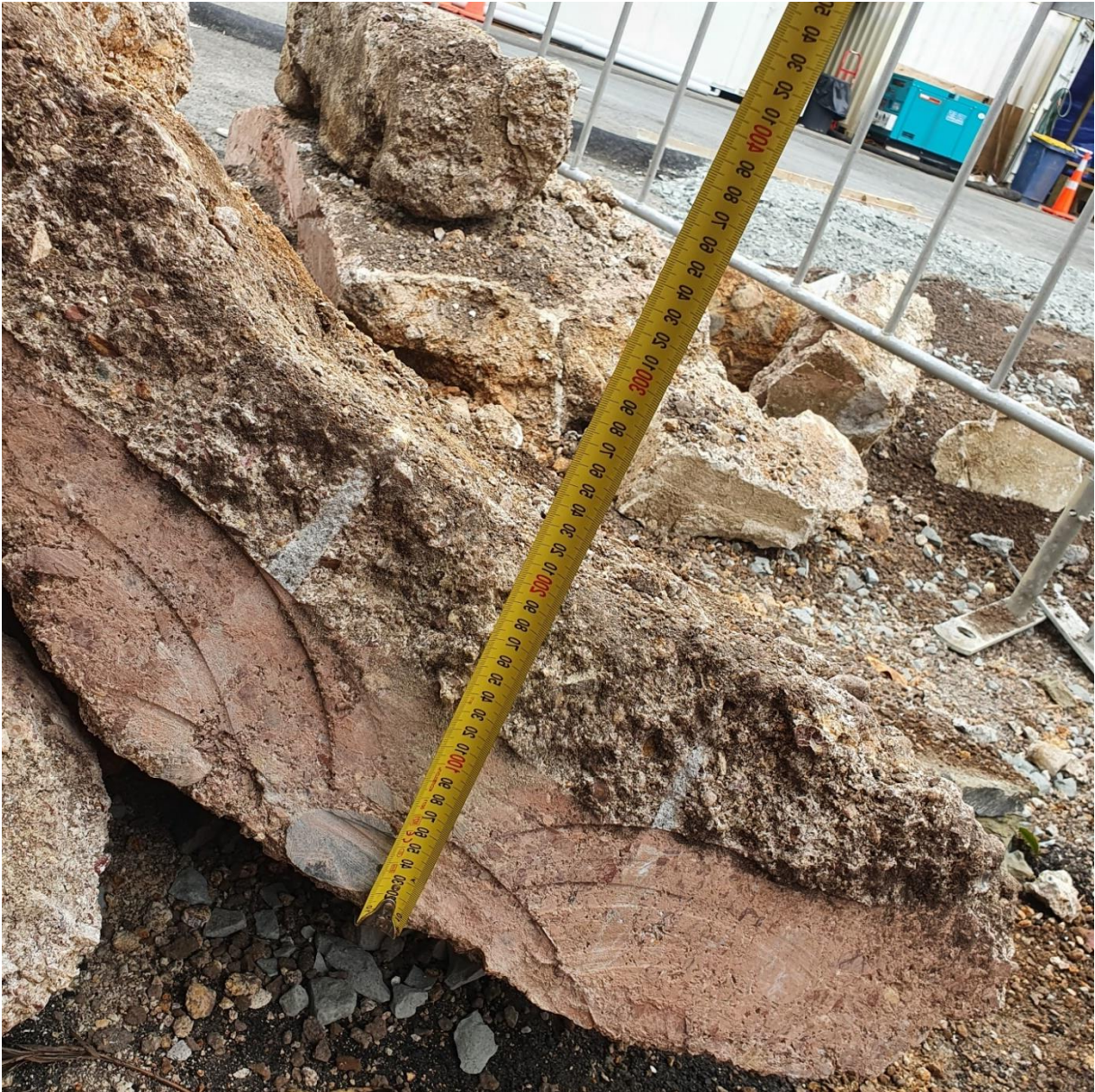
Figure 8 Weak blockwork after removal
