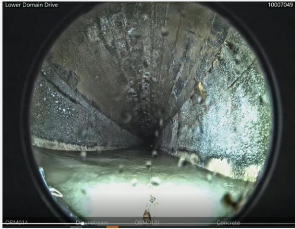
Mortar missing at 3 and 9 o'clock of CH: 222.94m
