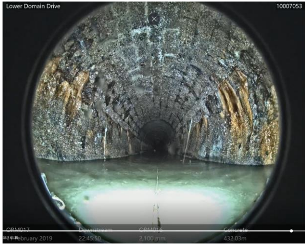
Dripping infiltration at 1 o'clock of CH: 432.03m
