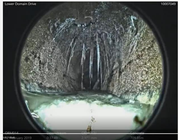
Tap root intrusion from 10 to 3 o'clock of CH: 709.85m
