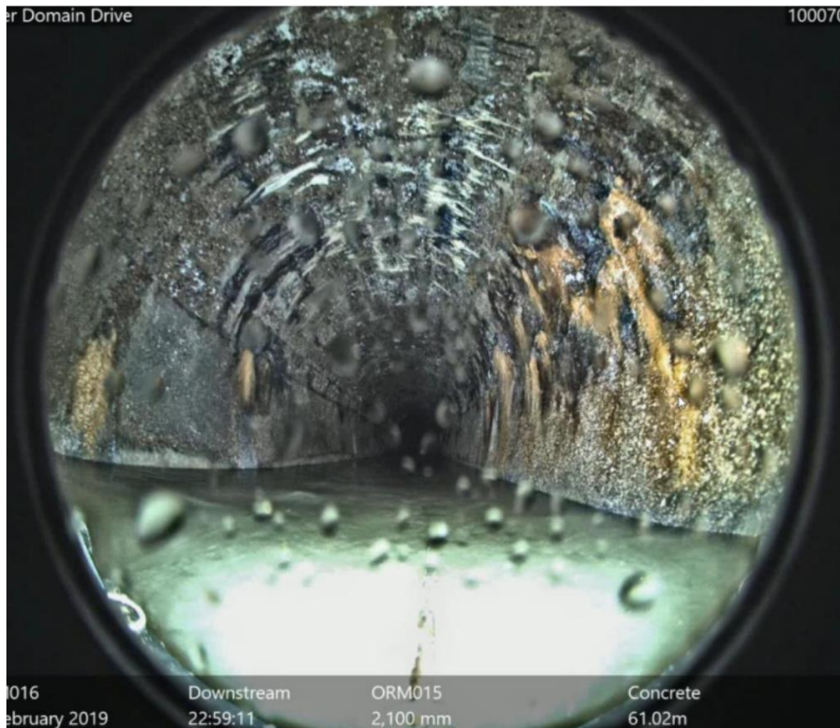
Figure 7.4 Sample CCTV output from OMS in 2019, shows the location near the collapse (supplied by WSL)
