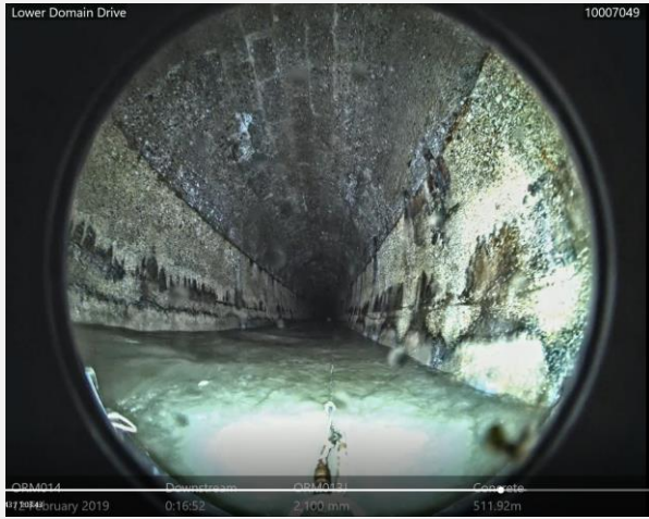
Mortar missing at at 4 o'clock of CH: 511.92m
