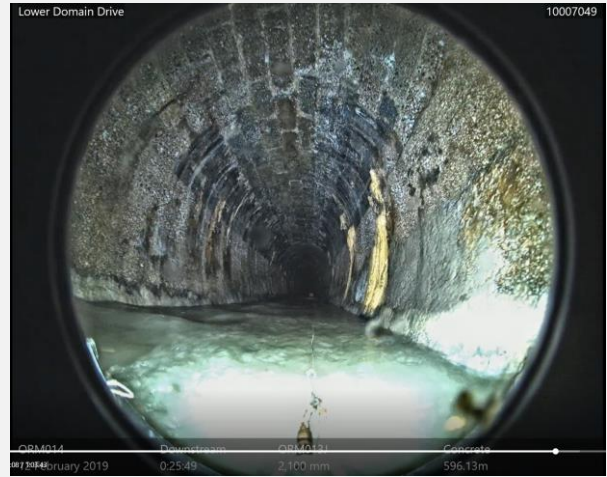
Dripping infiltration seen at the obvert of the pipe at CH: 596.13m and 598.23m
