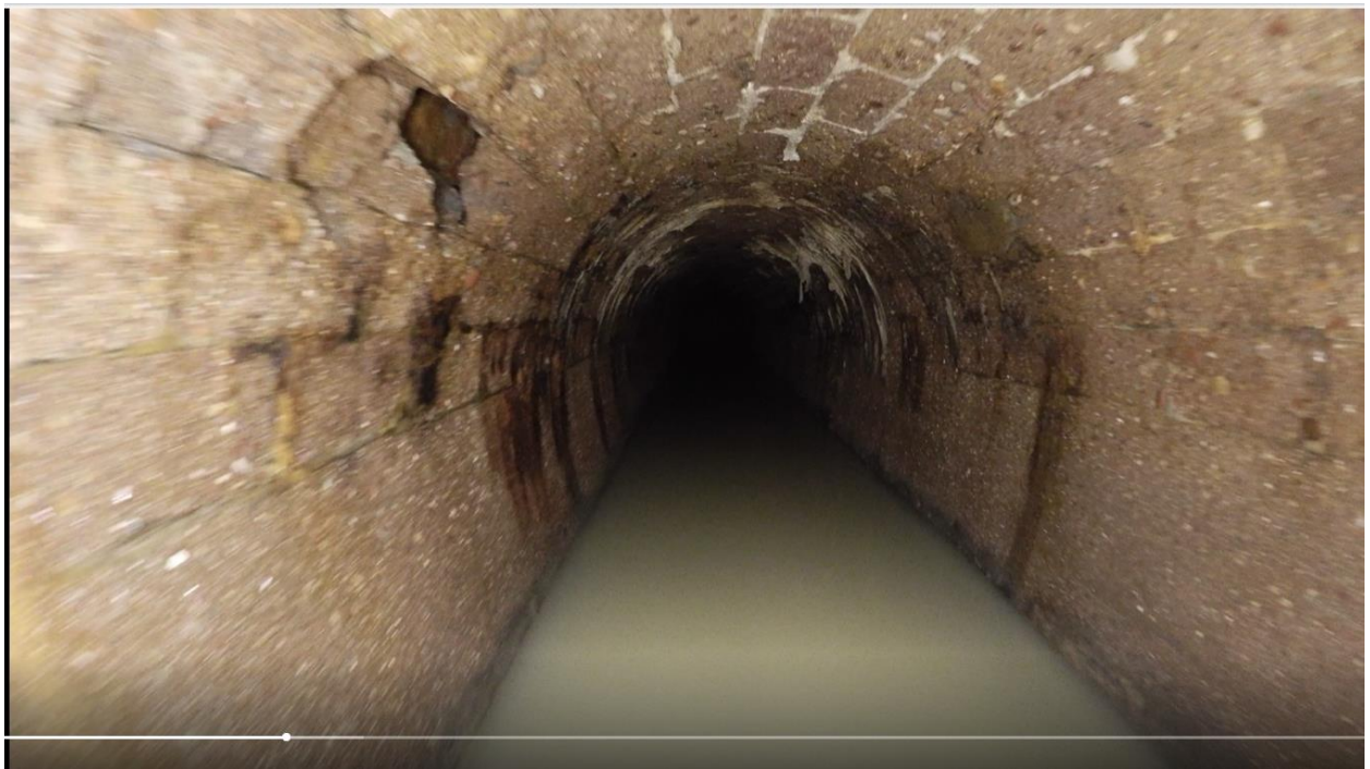
Figure 2 – Missing block between Manhole 15 and collapse (view is looking upstream, missing block is at 10 o'clock)
