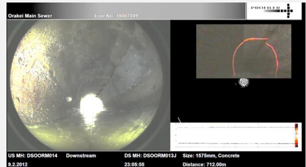
Longitudinal crack, assumed at mortar joint, observed at 1 o'clock from CH: 712m to 717.6m
