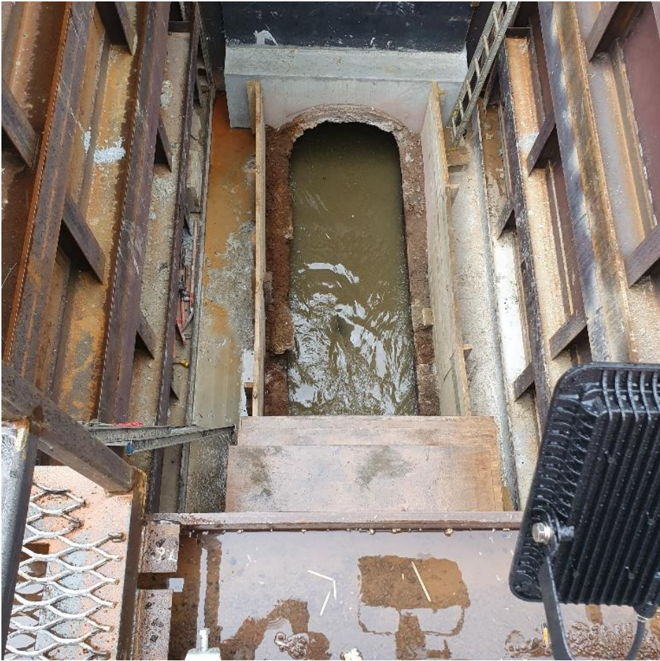
Figure 2 Looking down at OMS after installation of corbels and removal of block arch
