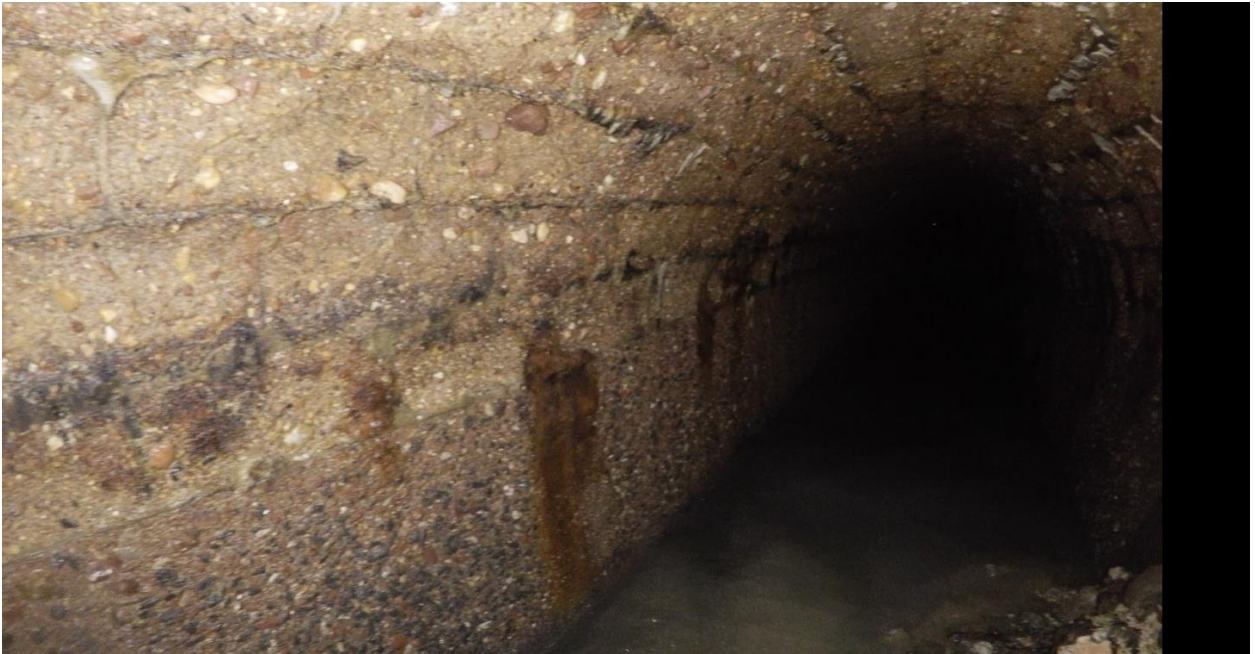
Figure 3 – View of Exposed Aggregate observed between Manhole 15 and the Collapsed Section
