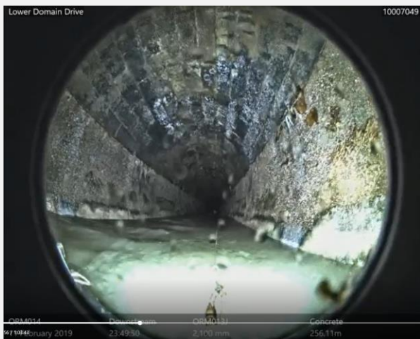
Mortar missing at 3 o'clock of CH: 256.11m
