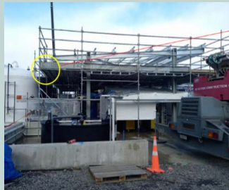
Scaffold toe-board plank loosens on this end.
