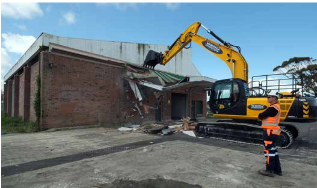
Demolition activities are underway at our Māngere site to prepare it for construction of shafts and pump station.
