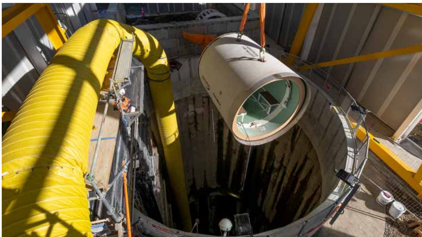
This photo shows the lowering of the first jacking pipe into our 55m deep shaft at May Road - another key milestone for the Central Interceptor project. The first pipe contains specialised equipment like our water cooling safety system. These pipes are lined with a 2.5mm thick layer of high-density polyethylene (HDPE). The HDPE layer protects the pipes from corrosion. In total 1097 pipes will be used to form the Link Sewer C tunnel running between May Road and Miranda Reserve.
