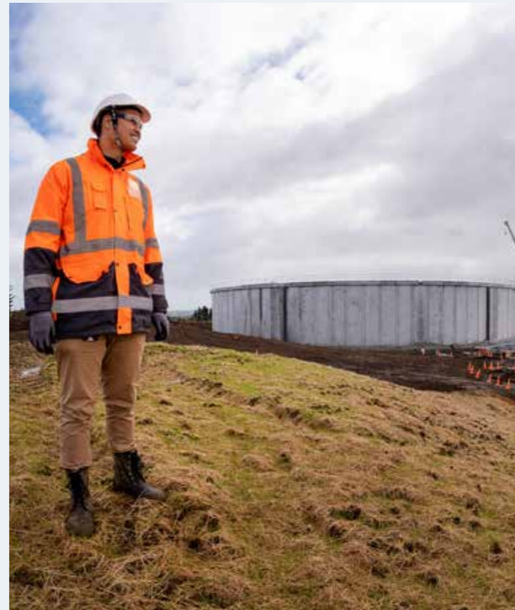
Project Manager Faiz Salim checks progress on the Pukekohe East Reservoir (concrete tank) in Runciman in July 2020.
