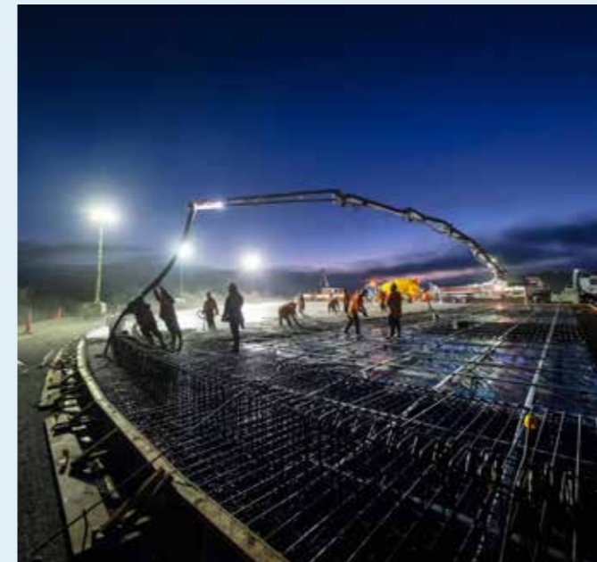
A convoy of concrete trucks recently delivered approximately 273 cubic metres of fresh concrete to our new Pukekohe reservoir site.
