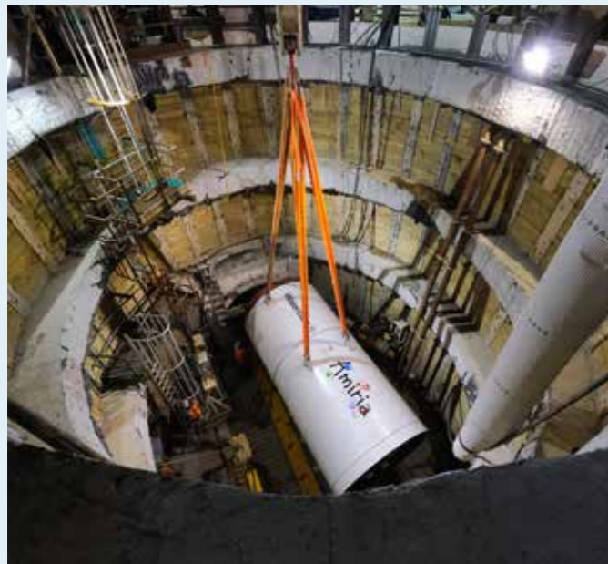
Our tunnel-boring machine called 'Amiria' is constructing the Hūnua 4 watermain. 'Amiria' is the te reo Māori version of the name Amelia and means hard-working or industrious.
