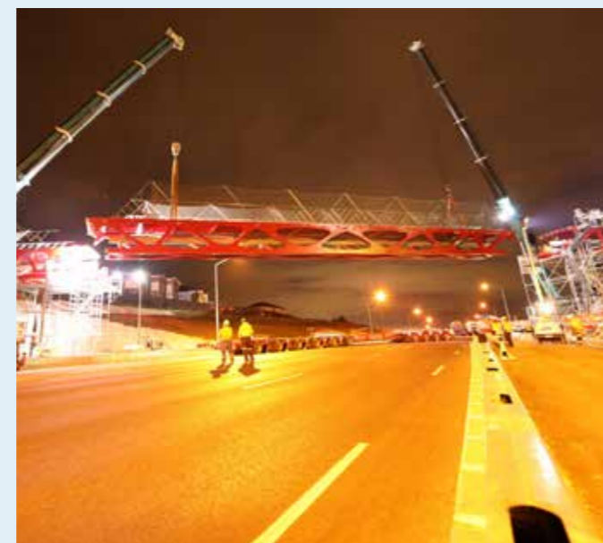
The Tirohanga Whānui bridge being installed. (Photo courtesy of the Northern Corridor Improvements Project.)
